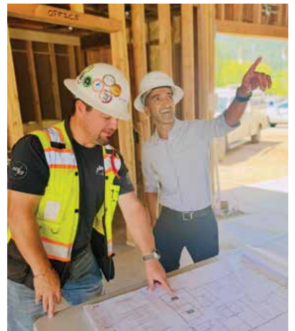
Dr. Raj Kalra, founder of Aroha Memory Care by MD Senior Wellness, reviews architectural drawings with Joel Ruiz of DesCor Builders at the construction site. The memory care center, located in Oakmont, is expected to open in late 2025. (Photo by Garrett Nichols)
